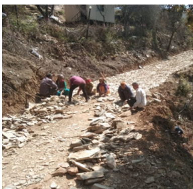
From top to bottom: Current state of classrooms, preparation of the site, parents preparing the road to the school
