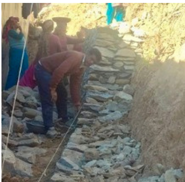
From top to bottom: New transitional school building, preparation and laying foundations of the retaining wall
